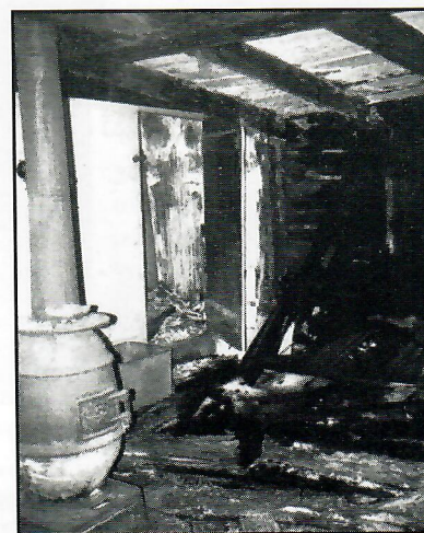
Half of the second floor had collapsed to the first floor. The exposed log walls are shown on the right side.
